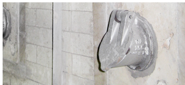
Melting tank superstructure/detail of peephole block
