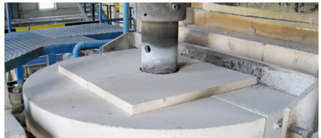
Spout area (burner and cover blocks)
