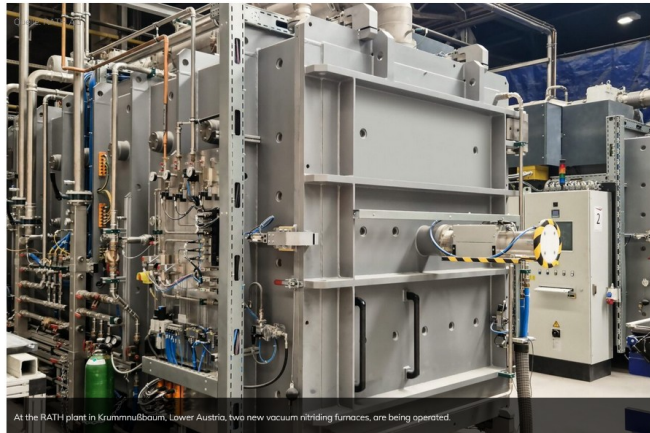
At the RATH plant in Krummußbaum, Lower Austria, two new vacuum nitriding furnaces, are being operated.
