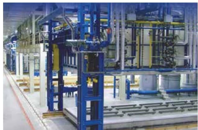
Bell-type furnace plant by CTB, lined with Altra modules, among others
