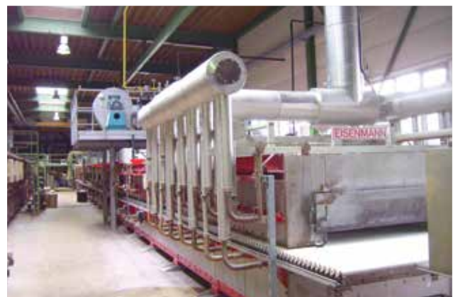
Roller furnace for annealing alumina mats
