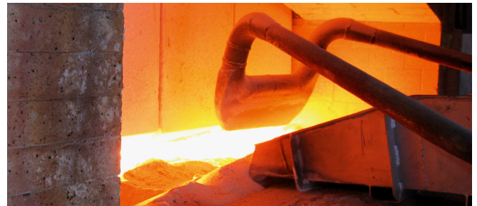
Melting tank superstructure/detail of peephole block
