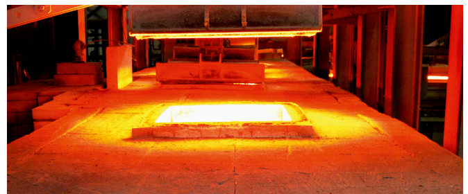
Distribution channel/forehearth superstructure insulation, with detail of flue openings
